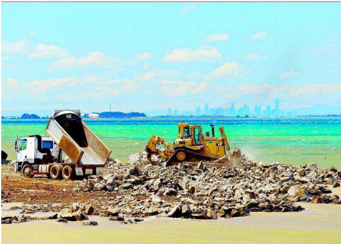
30,000 tonnes of rock being pushed into place as work starts at Wyndham Harbour.
